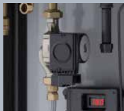
High Flow Recovery Pump
